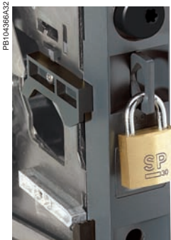
"Disconnected" position locking by padlocks.
